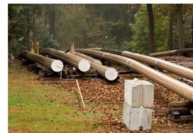
A pipeline under construction. An alert from the Department of Homeland Security shows the energy sector's vulnerability to hackers. PHOTO MATT ROHRKE/ASSOCIATED PRESS
